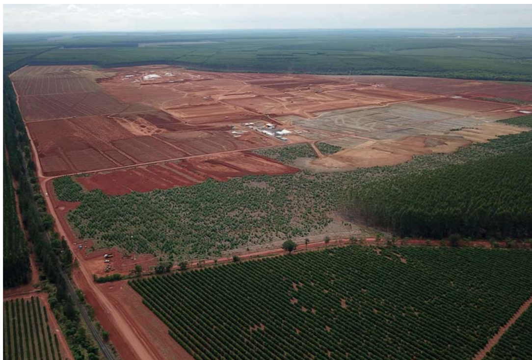
Site of the 500,000-tonne dissolving wood pulp mill being built at Minas Gerais state in Brazil
