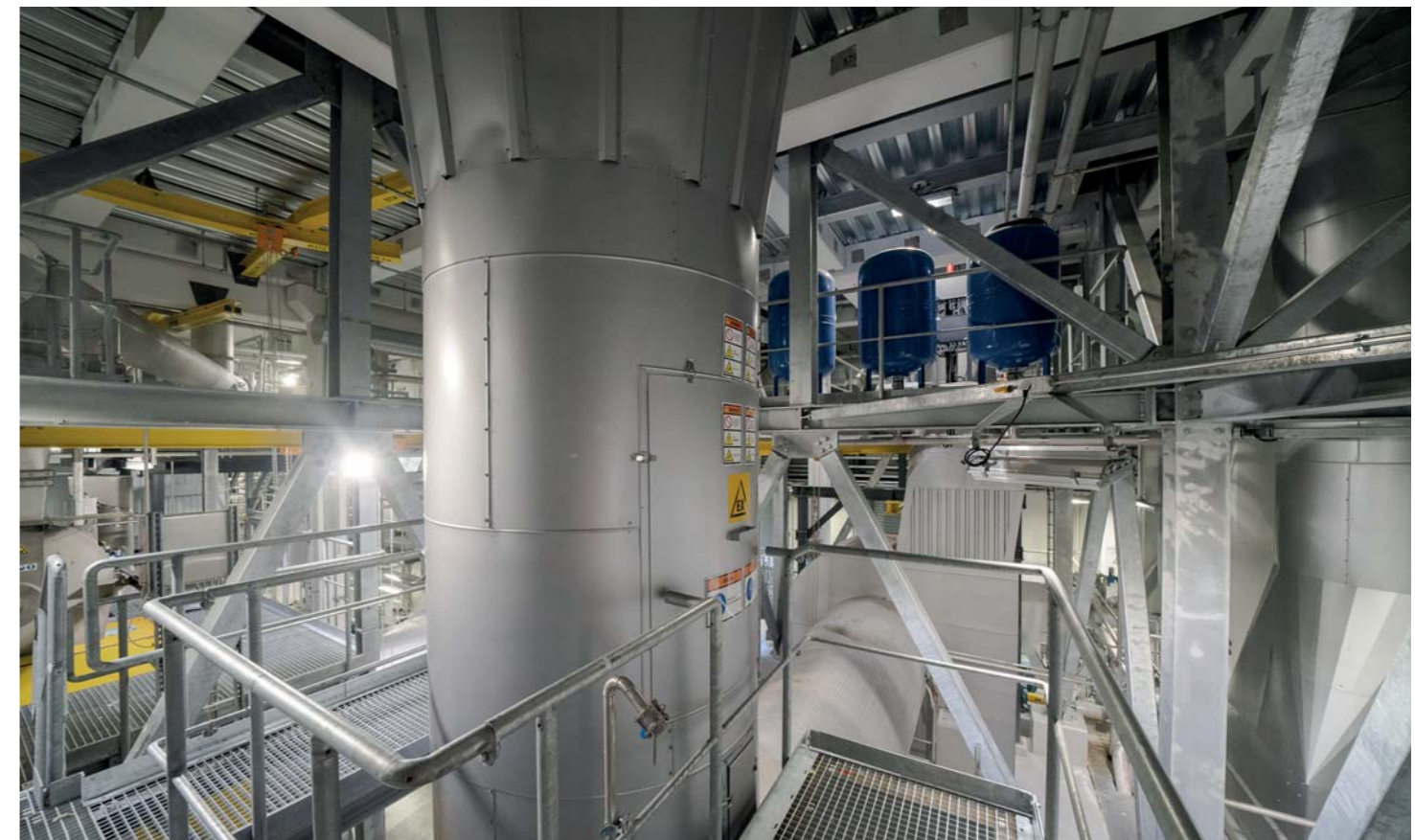
Equipment is easily accessible for service and maintenance, despite the tight space
