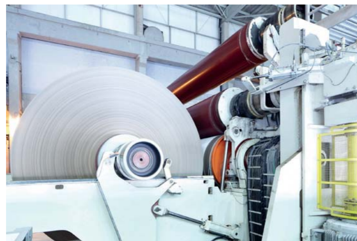
An understanding the health of drive systems means that the root cause of any paper machine problem is more easily resolved
