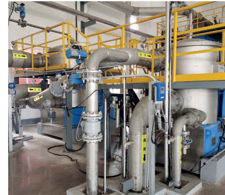
Two OCC lines have been delivered to Wamat Paper in China
