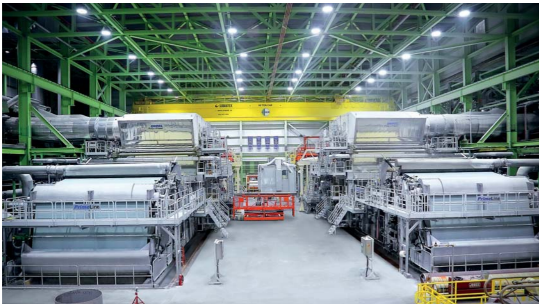
St Croix Tissue has successfully reduced variation in the final product using an artificial intelligence platform from Solenis
