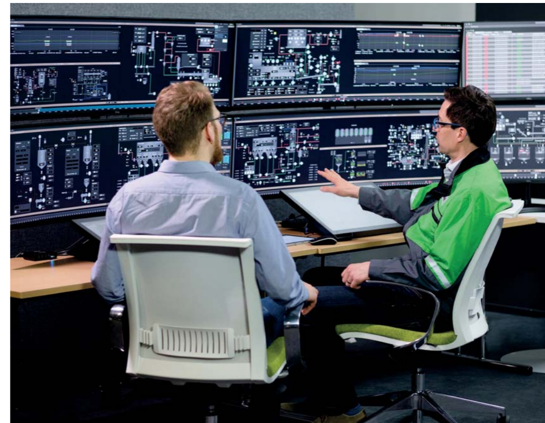
The control room set-up is transformed into a more transparent operation. Displays are arranged according to hierarchy levels, starting with the overview
